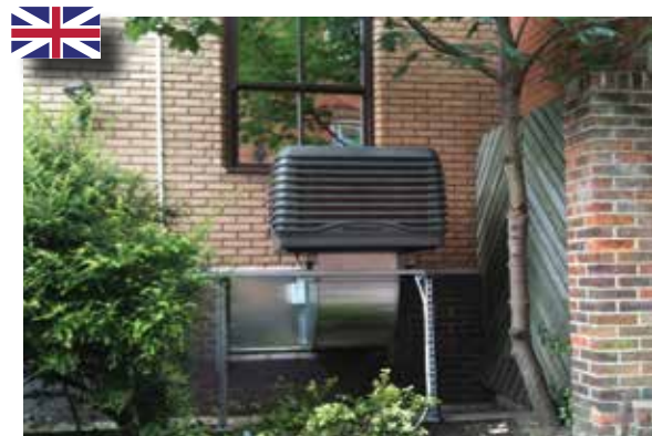
Datacenter UK | DATA CENTER
