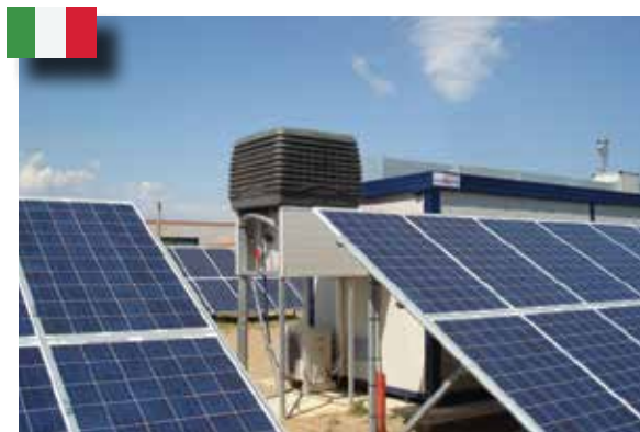
Solar panels Italy | SOLAR PANELS
