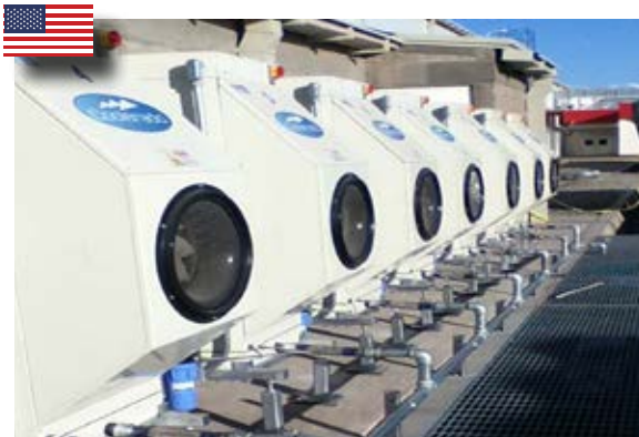
Kelloggs Cereal Processing Plant United States | Coolerado | Pre-Cooling
