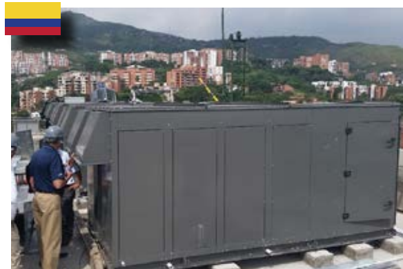
Centra Medica Imbanco Hospital Colombia | Coolerado | Stand-alone Cooling
